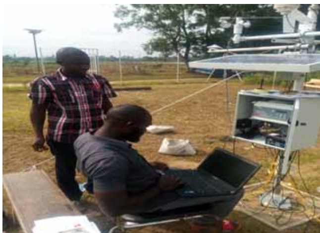
Installation and configuration of Data machine in Onna (Right)
